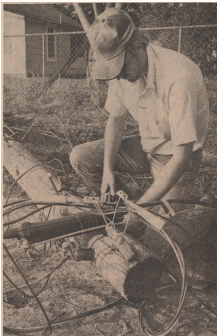
RESTORING SERVICE — Roger Honea, repairman with the Tri-County Telephone Company, works busily to restore telephone service to the more than 75 Garrison citizens who were without service Thursday evening as a result of telephone lines which were knocked down as a transport truck carrying an oil derrick through Garrison caught telephone and electric lines with its high load. The driver, William D. Reeves of Kilgore with the Big M Construction Company of Longview, said he was unaware of the accident, and the company has offered to pay for the damages, according to DPS Trooper James Moore. (Staff photo by Hardy Meredith)
